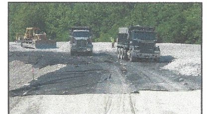
Figure 6 - Dump trucks carefully entering and exiting dumping points to prevent damage to fabric.
